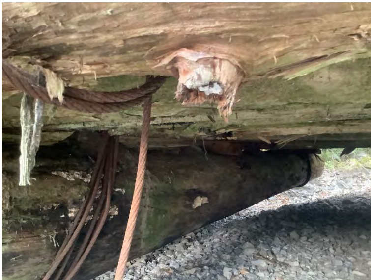
Needle beam, loose lashing not contacting stringers
